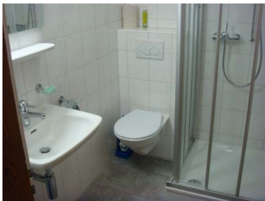
Figure 5: Part of the new sanitary facilities in the research station: shower room
