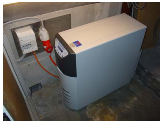
Figure 6: The new central UPS in the Sphinx laboratory
