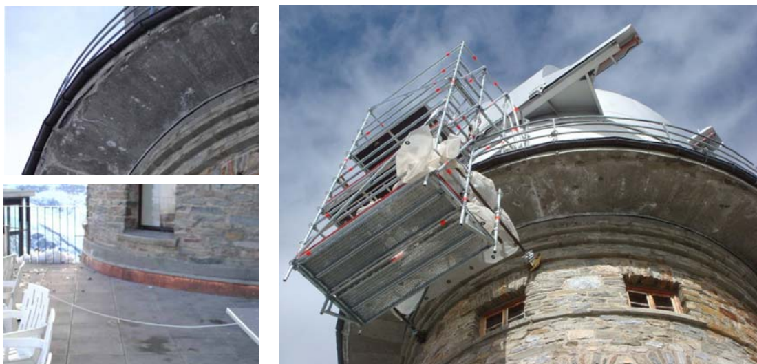
Figure 8: Structural damage and repair on the catwalk at the Observatory Gornergrat South.
