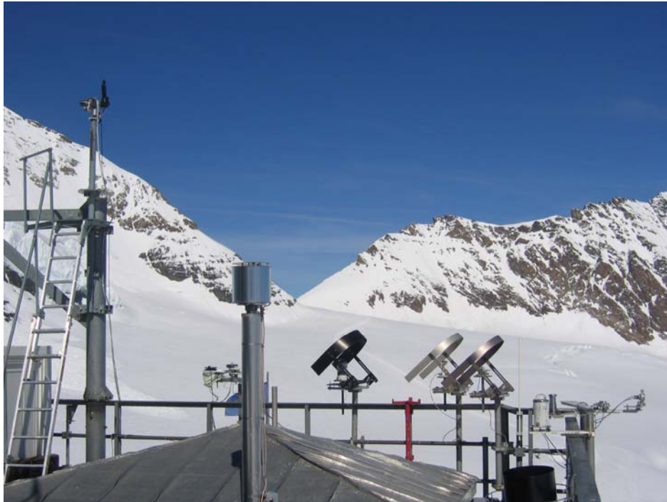
Figure 1: Installation of the radiation detectors on the roof of the Sphinx observatory, looking towards Mönchsjoch. On the right, detectors for global, UVA and UVB irradiance and in the middle the respective detectors covered by a shadow band to measure the diffuse component only. On the left on the pole the sun tracker with the input optics of the spectroradiometer for direct sun and diffuse sky measurements.
